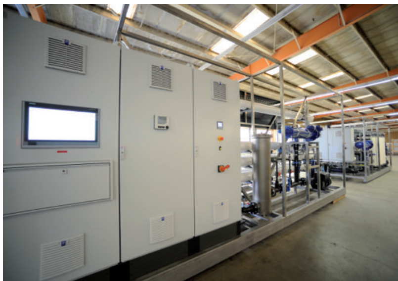
The plant is operated by a programmable logic control (PLC) with a touch screen interface, which is integrated into the frame of the reverse osmosis unit.
